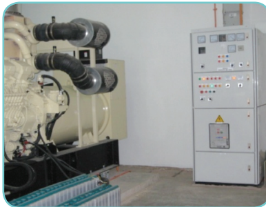
Naiktaraf kapasiti genset Hospital Melaka
